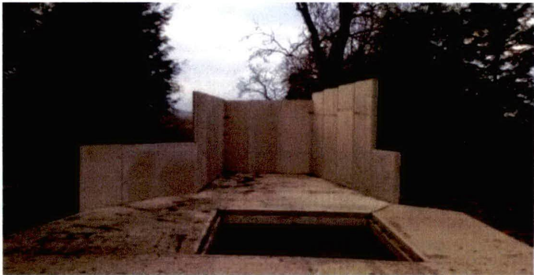
Muck store construction (central chamber to be covered with a grid when in use)
